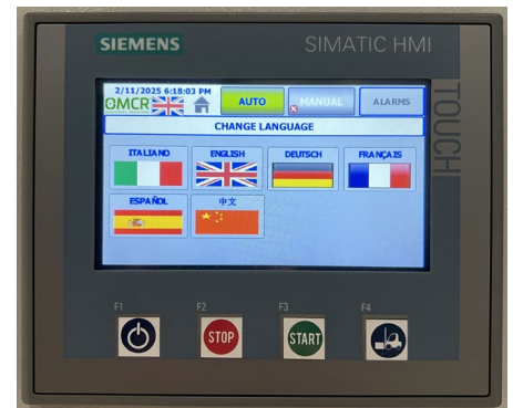
Control panel - detail
